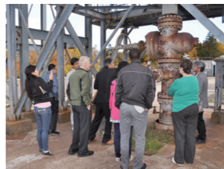
澄川地熱発電所の生産井 One of the production wells of the Sumikawa geothermal power plant
